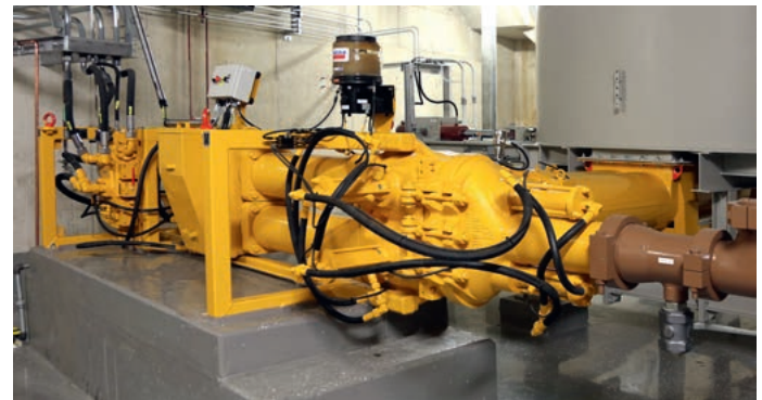
WWTP Buchenhofen, Wuppertal, Germany
